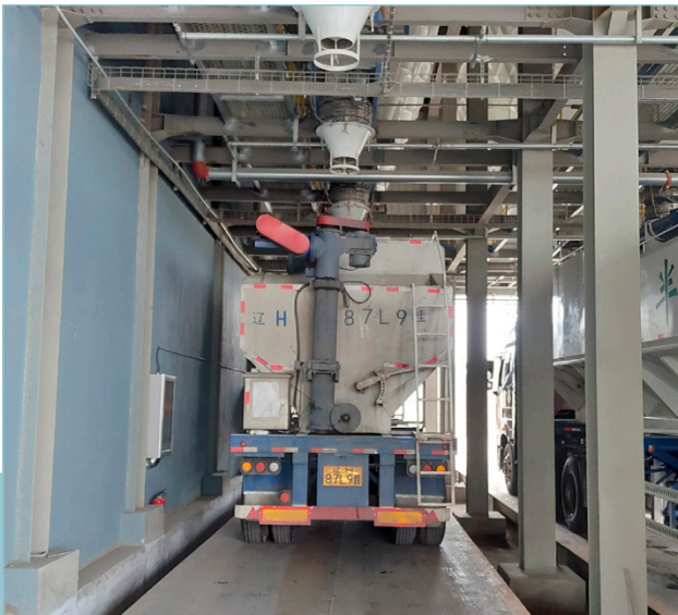
Efficient weighing and filling processes are key at New Hope Group’s discharge station
