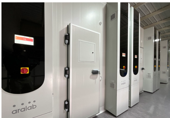
STABILITY ROOMS TURNKEY PROJECT BY ARALAB
