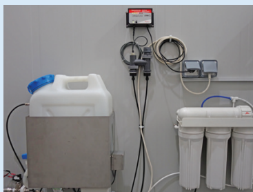
Water treatment systems
