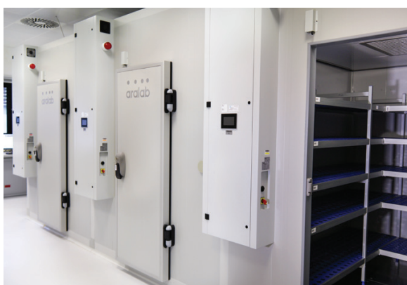
STABILITY ROOMS TURNKEY PROJECT BY ARALAB
