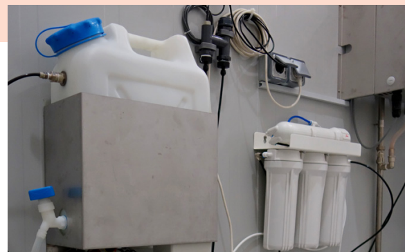
Water Treatment systems
