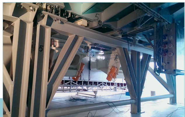
Six load cells were installed under each silo, with capacities of up to 75 tonnes
